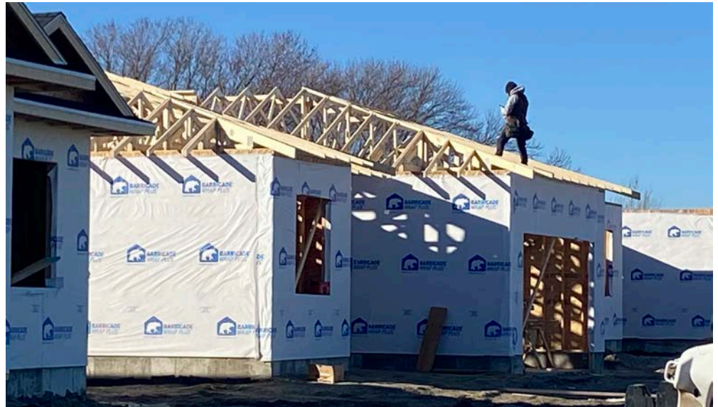
Workers found the early December warm temperatures conducive to house building in the new Northern Meadows subdivision in Holdrege.
