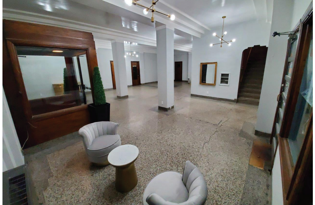
Renovations on the historic Hotel Dale (now called The Dale Residences) have started as the property was purchased by new owners in September. Renovations could take a year. Photo Courtesy of Melissa Ann Wills.
